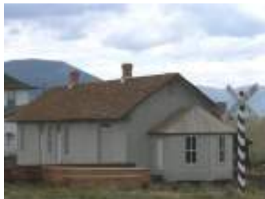
Above: Como Depot on July 27, 2014. Older than Dirt Construction company began the final phase in summer 2013 and expects to finish both the exterior and interior by the end of August 2014. Stay tuned!
