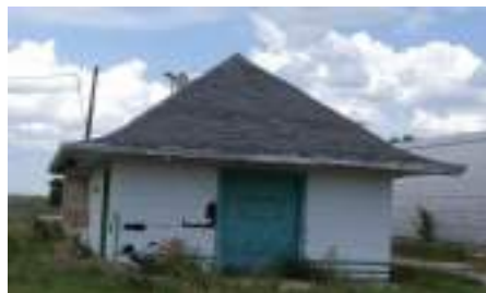
View of west side of depot showing some subsidence
